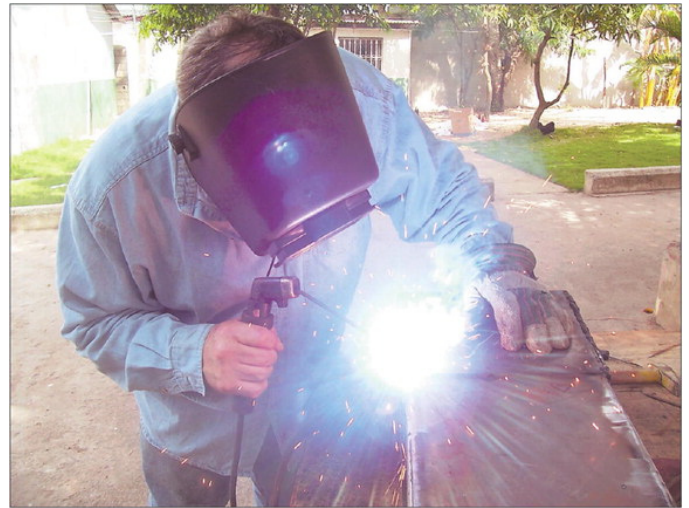
Tom Oppelt of Wallingford works on a water filtration system in La Romana.
